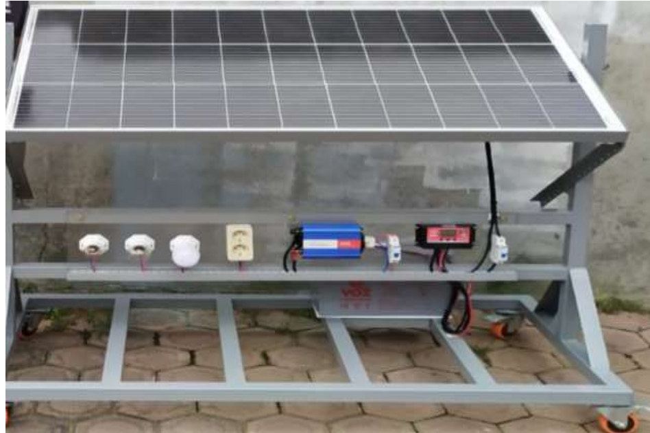
Figure 1: Simply solar power plant
